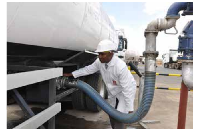
A Kenya Pipeline Company employee displays a bottom loading facility at KPC Eldoret Terminal. Over and above ensuring safety through minimal spillage of petroleum products, bottom loading facilities are a major milestone in the petroleum industry's environmental sustainability evolution owing to reduced air emissions. KPC is marking 50 years since establishment in 1973.
